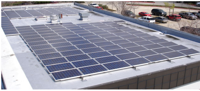
Fig. 1. PV installation on a flat commercial rooftop in California (using SunLink LLC's first generation of non-pervasive mounting system).
